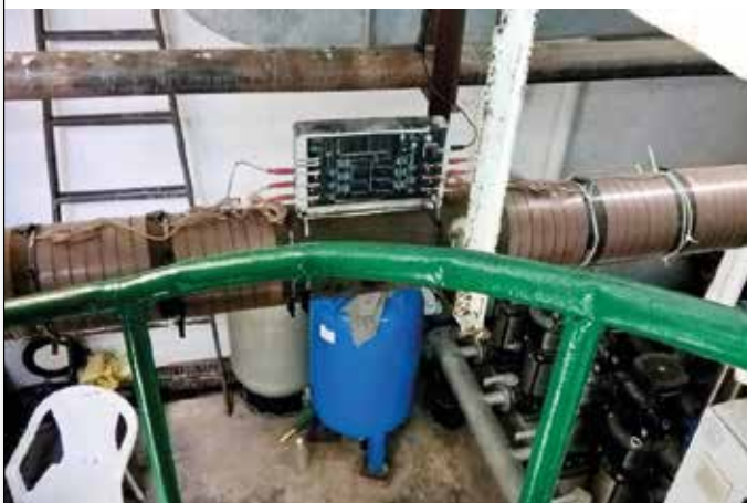
Two Vulcan S100 were installed.
