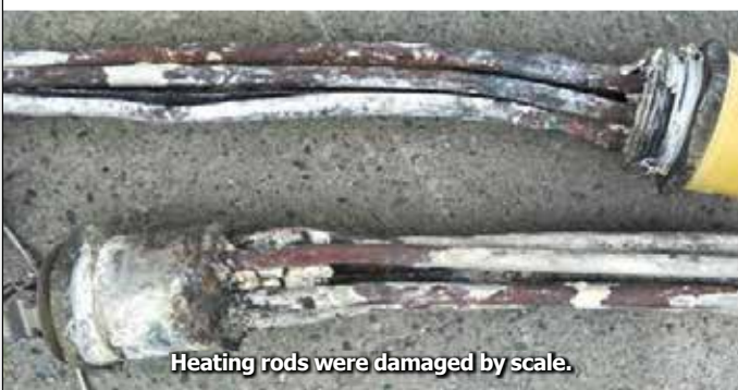
Pipe joint fittings had to be replaced because of scale and rust.
