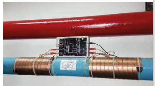
Anti-Scale System Vulcan S25 installed
